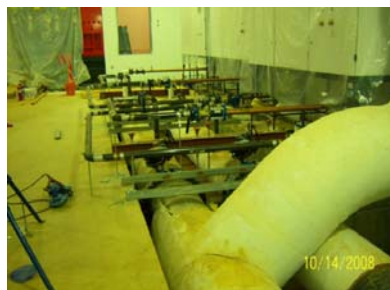
Figure 1 - Mechanical trench in a computer room.
